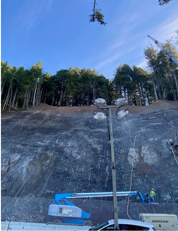
Caltrans crews used mesh anchors to shore up the hillside at Last Chance Grade. Photo courtesy of Caltrans District 1
