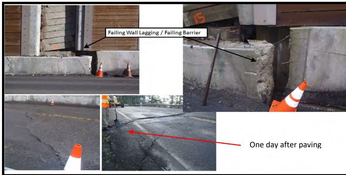
Figure 1. Recurring Damage Along Last Chance Grade 2
